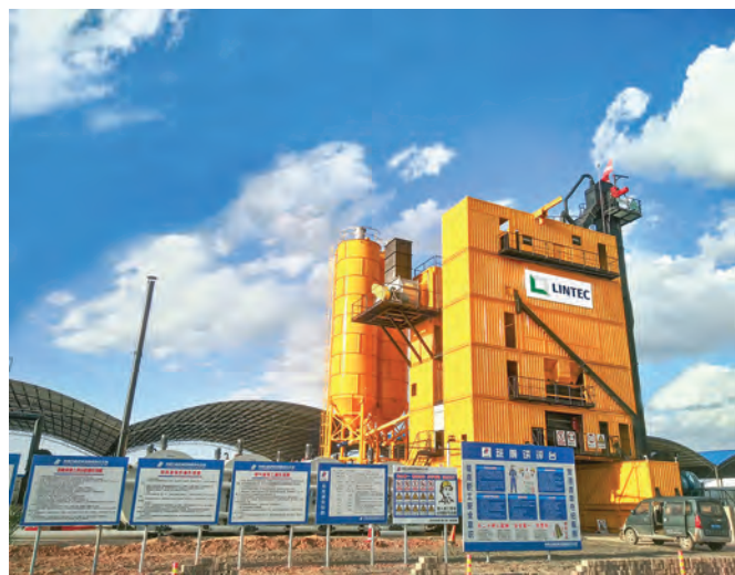
The Lintec CSM5000 asphalt plant worked on the 26-km-long G65 BaoMao Expressway before moving on to the construction of the Jingwu Expressway.
