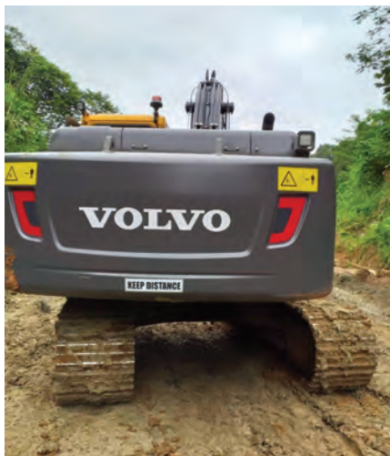
A Volvo excavator handles the muddy terrain at RFB Construction Company's site in Bukidnon province with ease.
